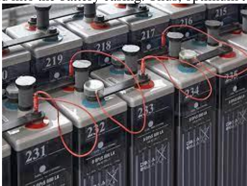
Fig 8. Battery Temperature sensor
